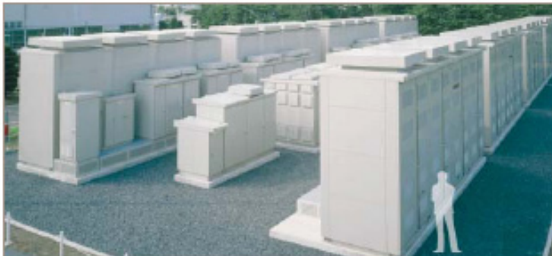
Fig. 9. NGK-supplied 9 MW, 57 MWh sodium-sulphur peak-shaving battery for Hitachi—one of the largest energy storage batteries in the world (source: Hitachi/NGK)
