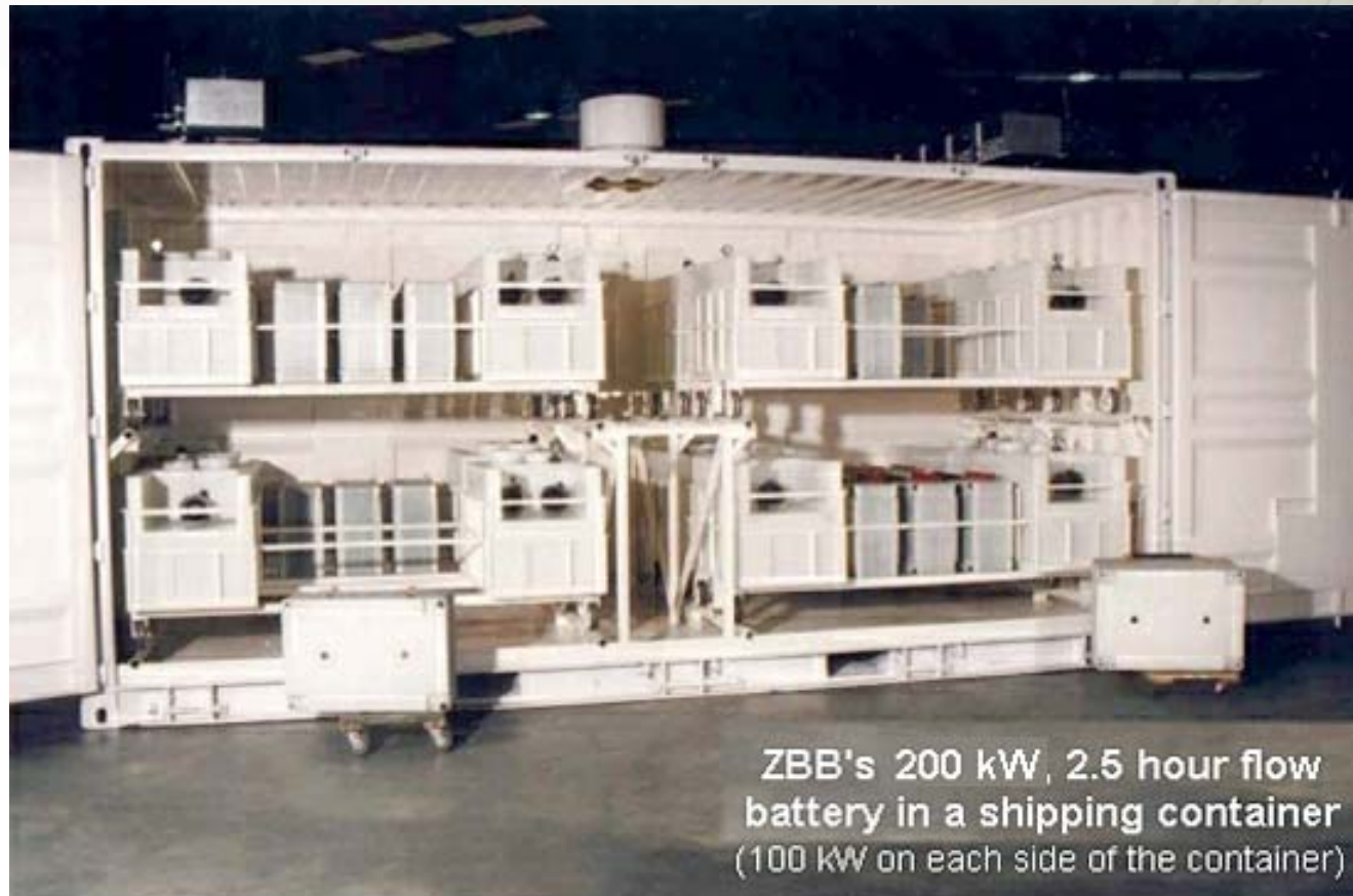
Photo Courtesy of ZBB Energy Corporation
